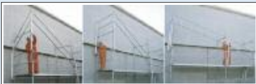
Example of an advanced guard rail system
